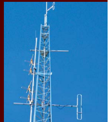
Typical antenna install on a Titan tower
